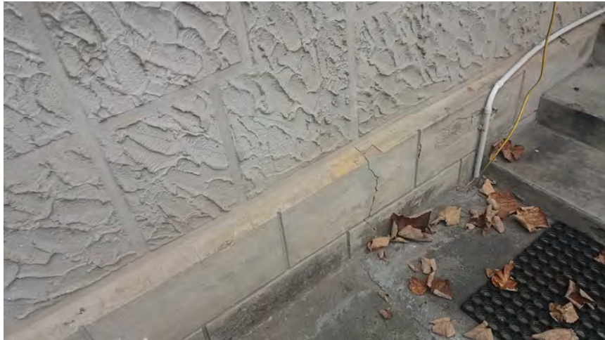
Discussion of Assoc. Prof. Dr. Claudiu Sorin Dragomir, Secretary General of ECBR with a lady owner a small house with cracks at socket, about the possibility to rehabilitate and add one attic as living space, delivering an ECBR leaflet
